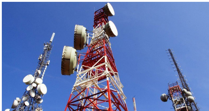
Mexico started an overhaul of its telecommunications sector a decade ago. Telecommunications towers in Mexico are pictured. // File Photo: Mexican Government.
